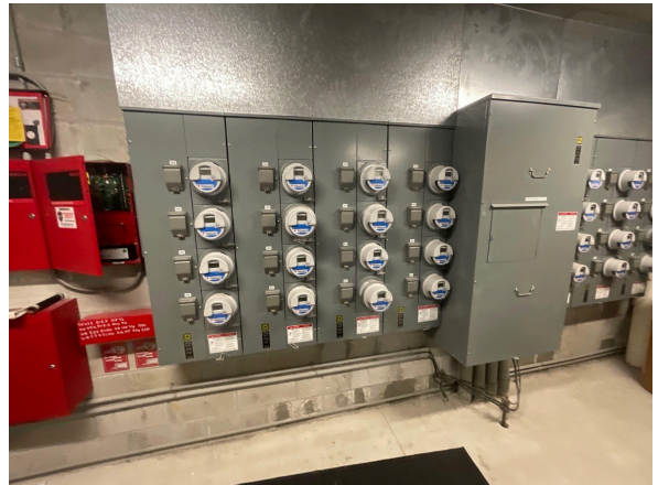
Typical electrical equipment
